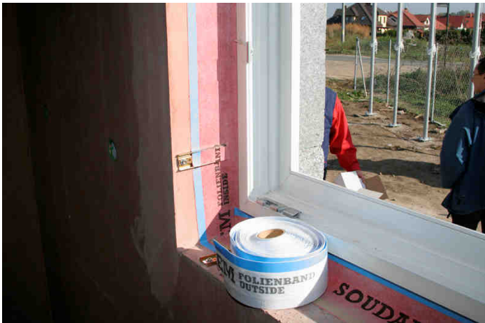
Drawing 7. Tight connection of external walls with the window woodwork – vapour-proof plastic wrap before gluing
